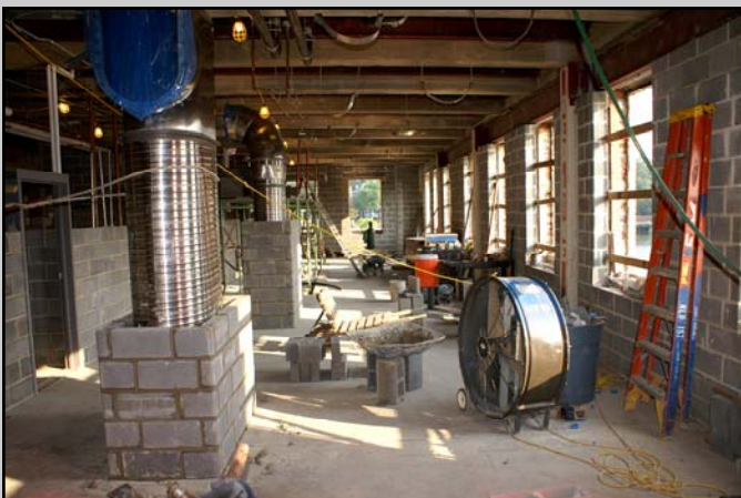
Men's Locker Room and New Ventilation System
